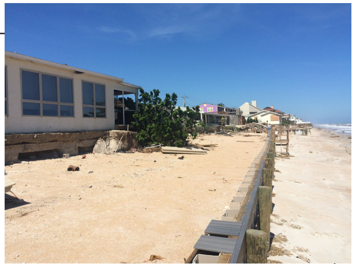
Coastal armoring cuts off the upper portion of the beach, causing sea turtles to lay their eggs in less optimal locations closer to the water.
